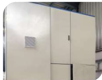
Zero Liquid Discharge Plant
