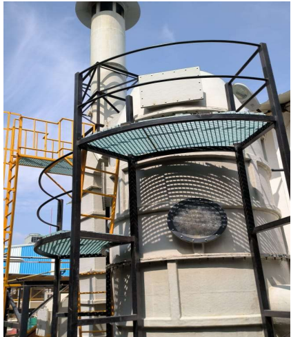
Air pollution control equipment
