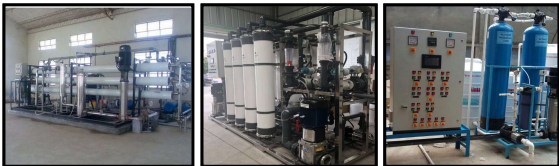
Effluent Treatment Plant
